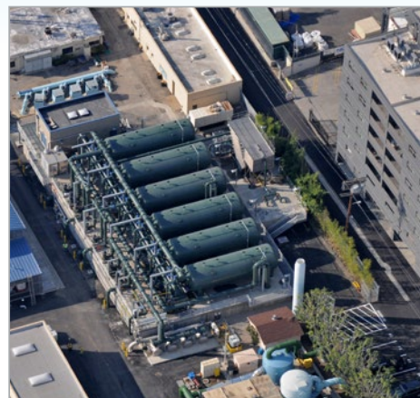
Horizontal Pressure Filters at Bundy Well Site
