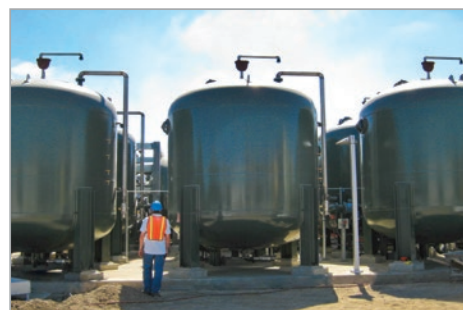
Vertical Pressure Filters at Westminster Well Site
