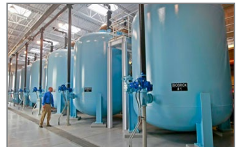
Magna Water Treatment Plant in Operation
