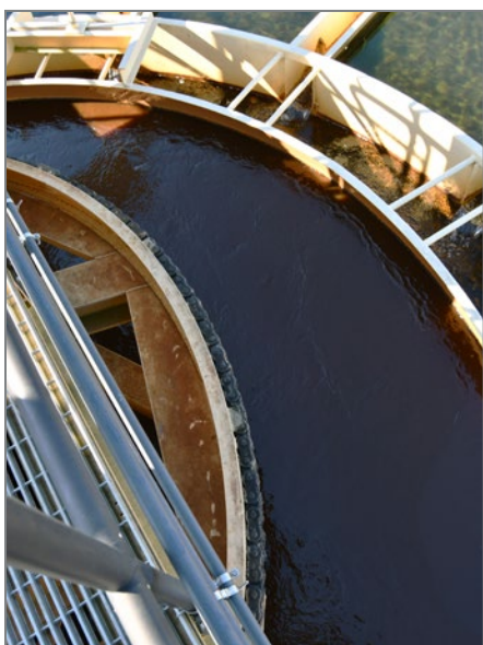
Newly painted CONTRAFLO unit installed in 2005
