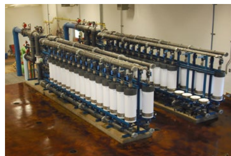
Ultrafiltration Membrane Filter Trains
