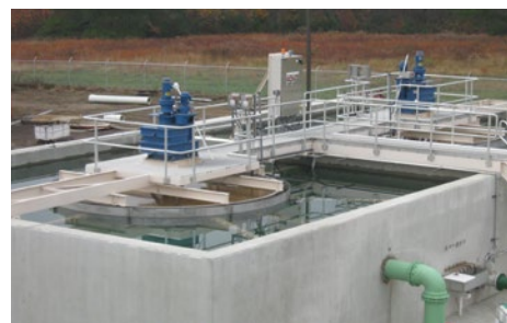
Solids CONTACT CLARIFIER™
