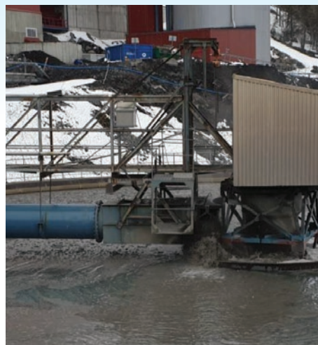
The small feedwells allowed foam to collect on the thickeners' surface from unsettled fine particles.
