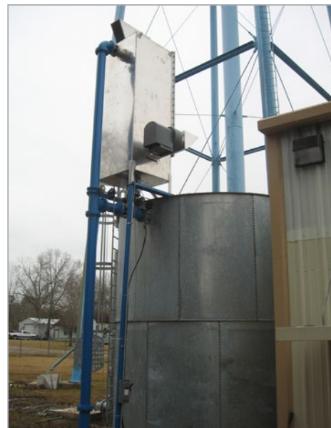
Forced Draft Aerator
