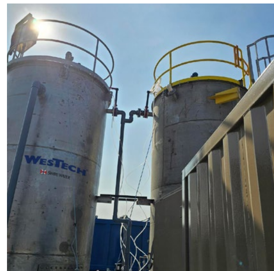
WesTech Solids Contact Clarifiers placed in front of the evaporators to remove solids buildup and enable a continuous process.
