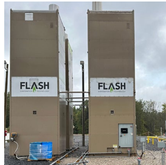
Four FLASH units were temporarily deployed to manage evaporation issues and stabilize pond capacity until the full systems were online.
